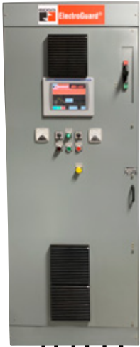
Main Control Panel (MCP) (MCP shown is a free standing, MCC-type enclosure.)
